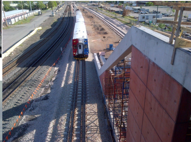
Stem walls and escalator in place for transfer station at North Temple
