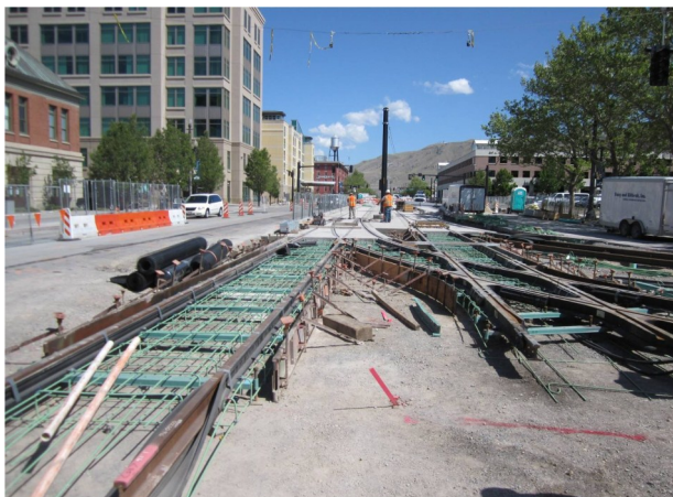
Tie in track work joins the Airport Trax Line with the existing line.
