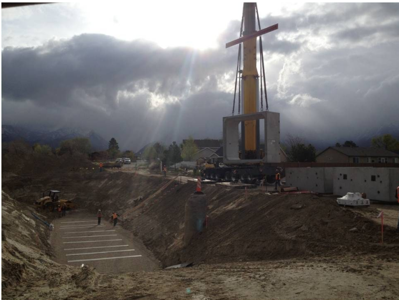
Installation of a tunnel for a planned horse trail in Sandy City
